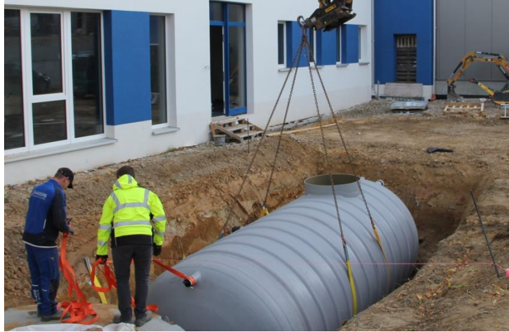
Picture 3: Fibreglass storage tank
