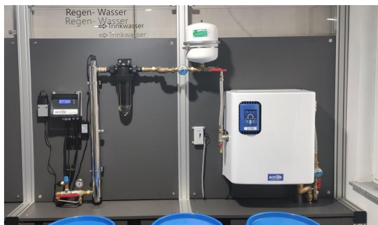
Picture 2: Drinking water treatment system
