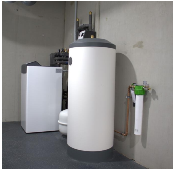
Picture 8: Central heat pump
